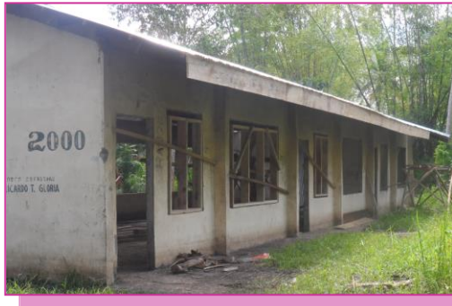
A school building in Barangay Gawang damaged by armed conflict
