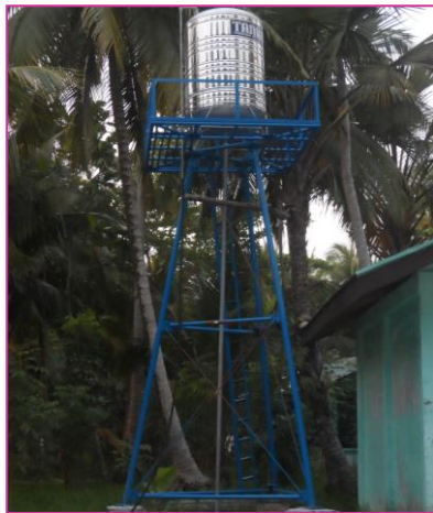
Level 2 water supply system installed in Barangay Gawang
