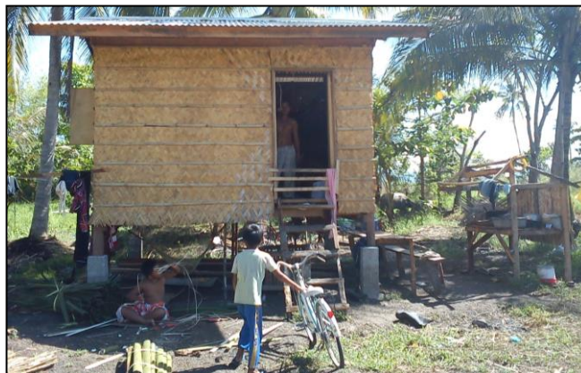
From the original shelter repair assistance to the construction of core shelter unit with 10x12 ft. dimension
