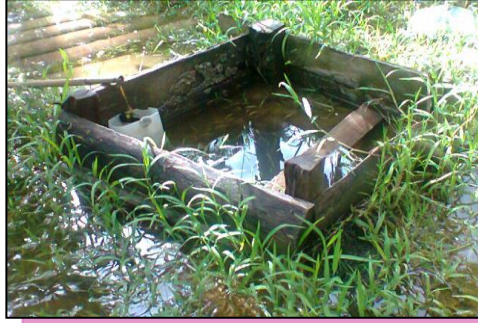
One of the dug wells affected by flood
