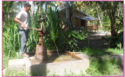
Level 1 water supply system installed in Brgy. Gawang
